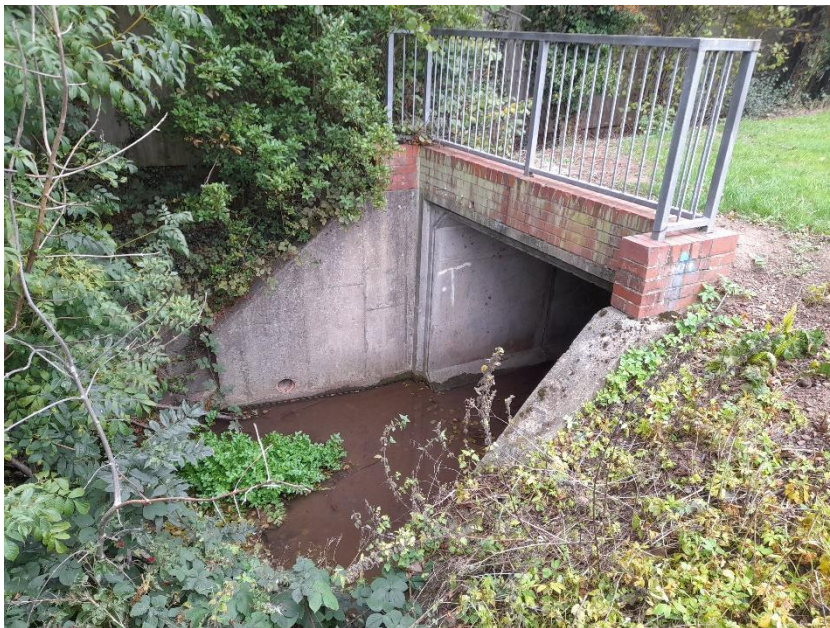
Culvert downstream at SP 29235 80507 (before it gets sandwiched between the two sides of the A4114)
